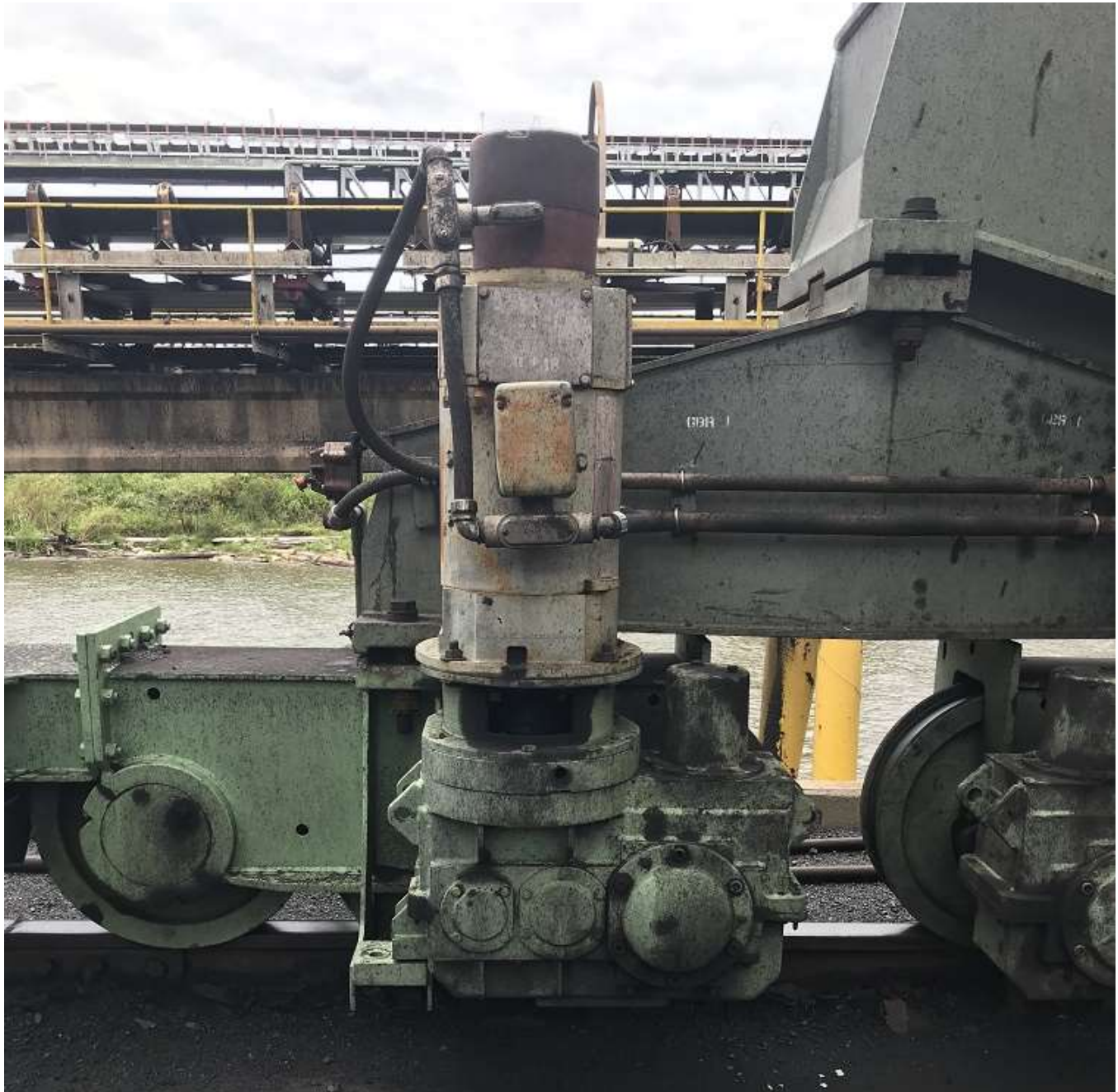
Flender Gearboxes for SL2 Gantry
