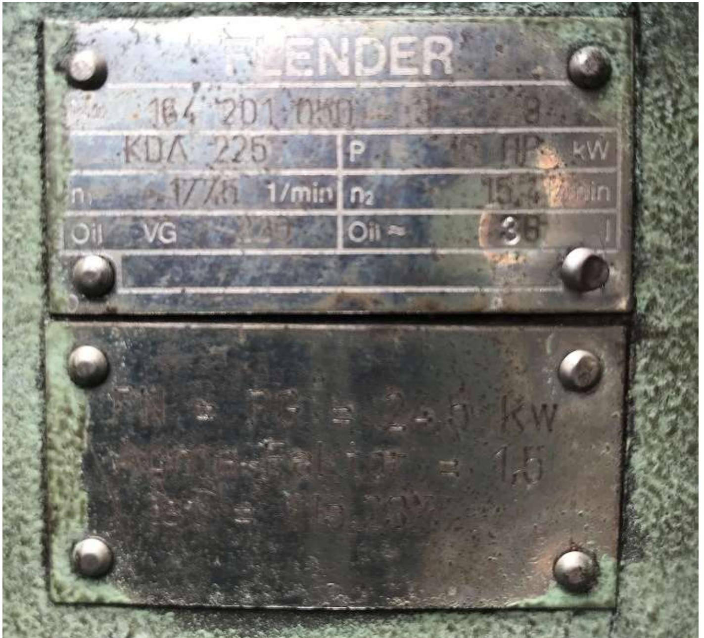
Flender Gearboxes for SL2 Gantry
