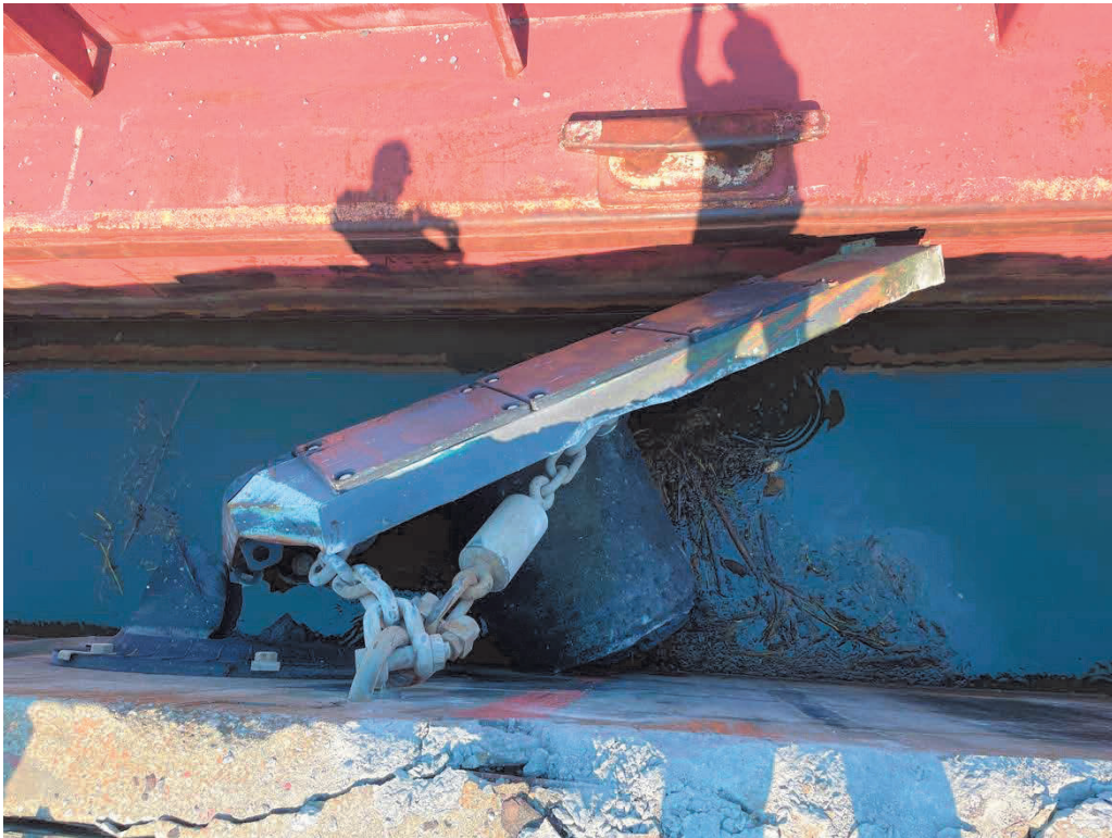
Damaged fender hanging from pier
