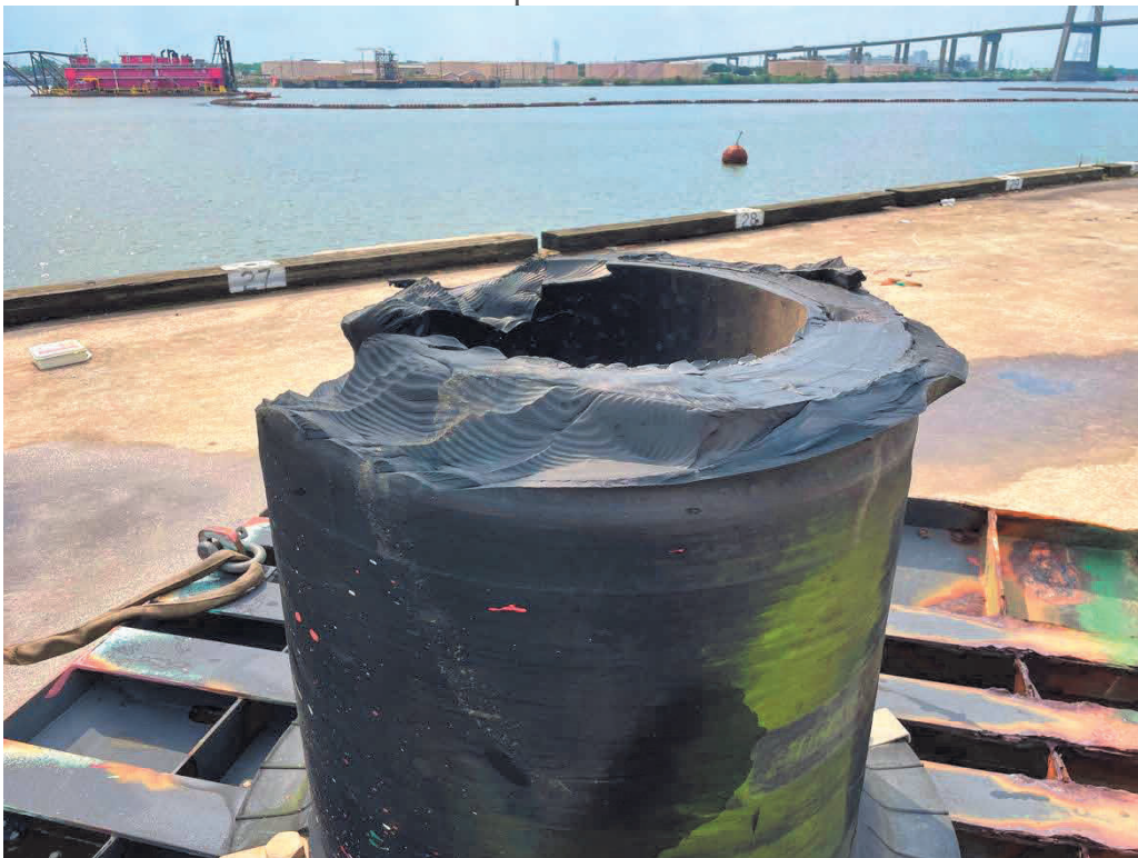
Rubber Element torn
