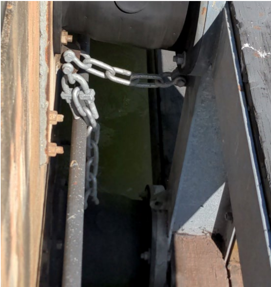
Example of broken chain to be replaced between bollards 8-9 or 12-13 - Bid Additive
