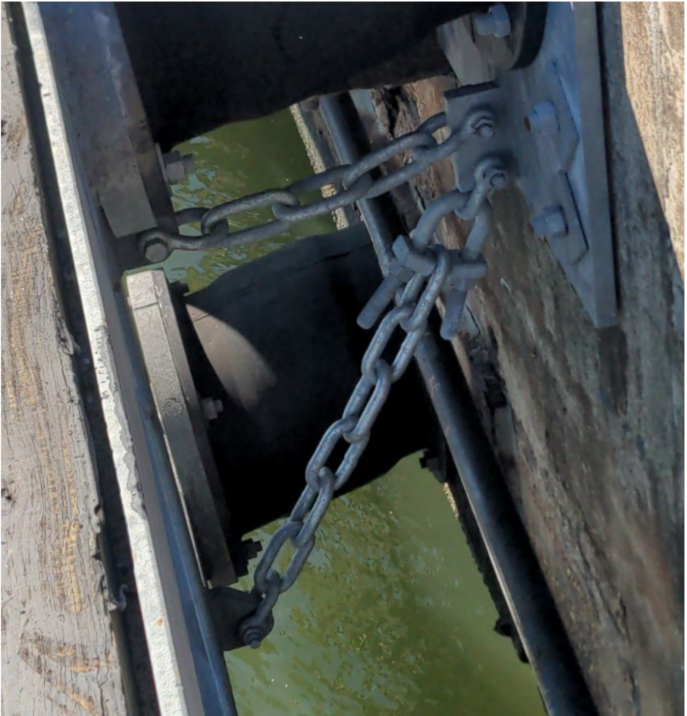
Example of single adjustable shackle to be replaced between bollards 8-9 or 12-13 - Bid Additive
