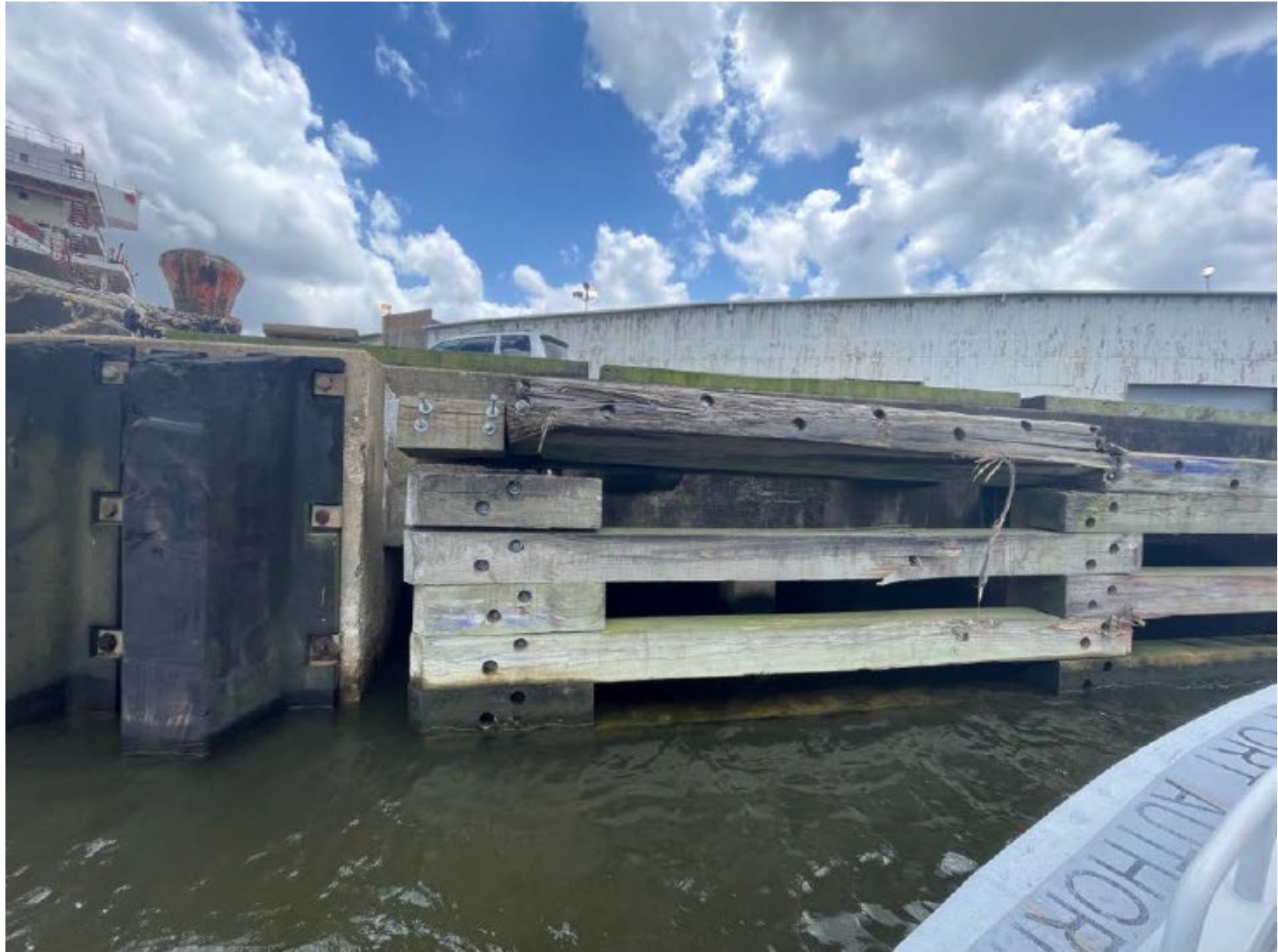
River view of damaged wale fender system
