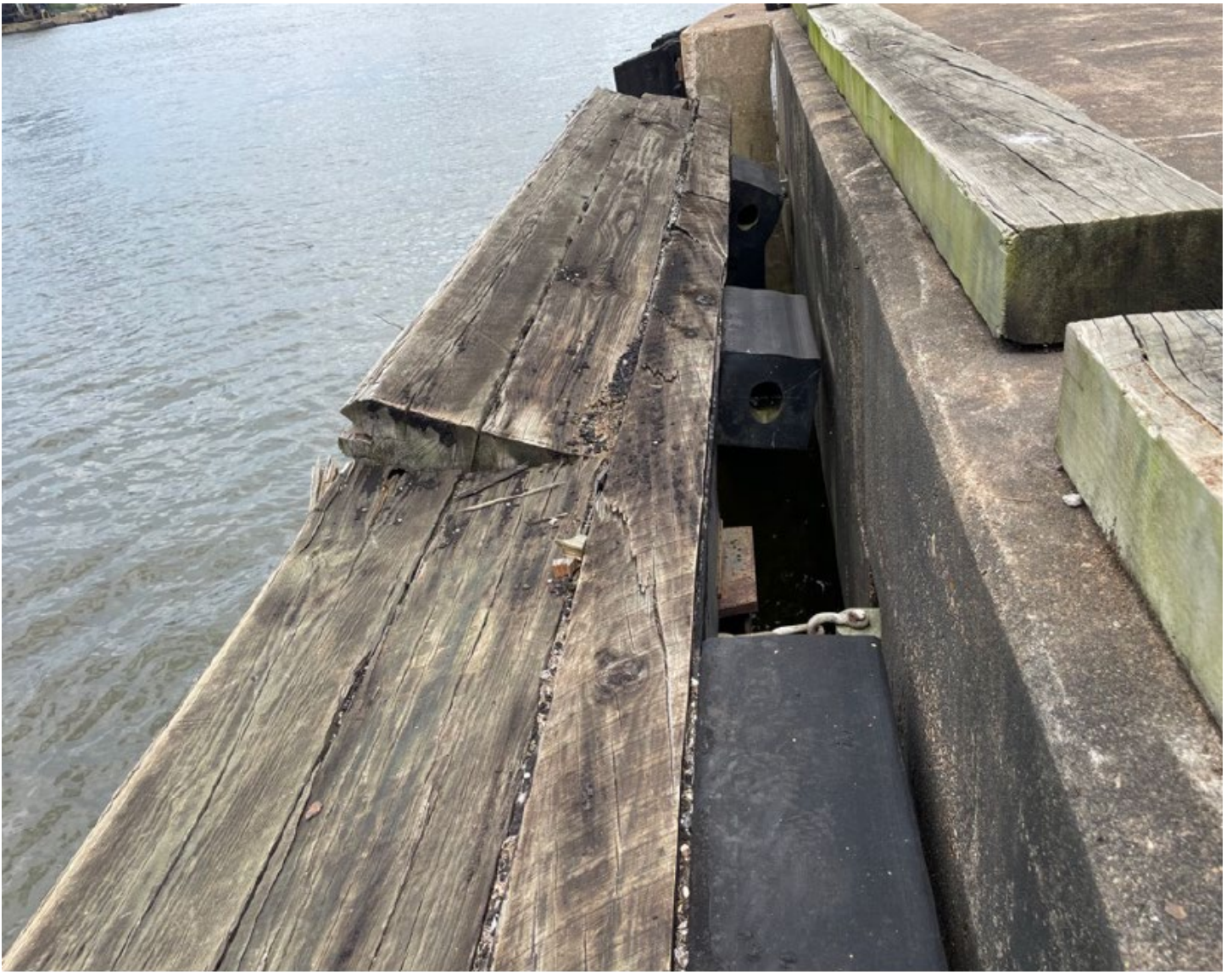
Note the cracks in the 6"x8" timber that sits in the steel wale
